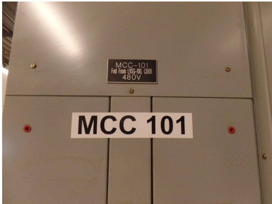
MCC 101 Name Plates
