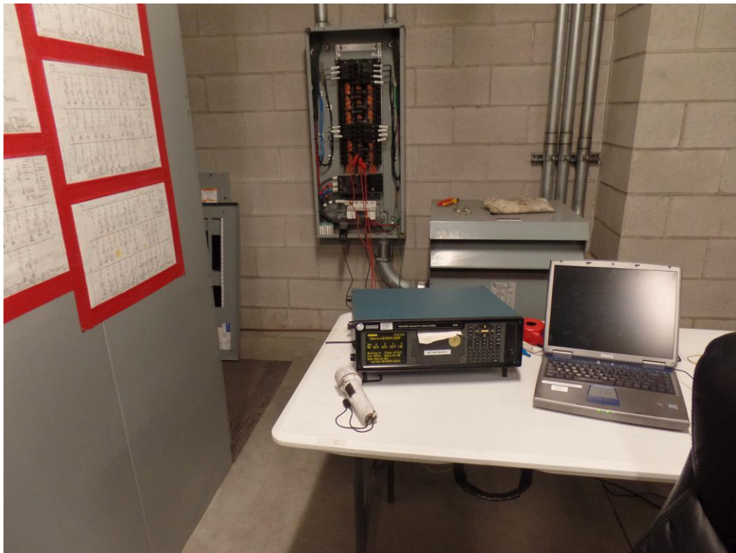
Test setup for Power Panel PP--102
