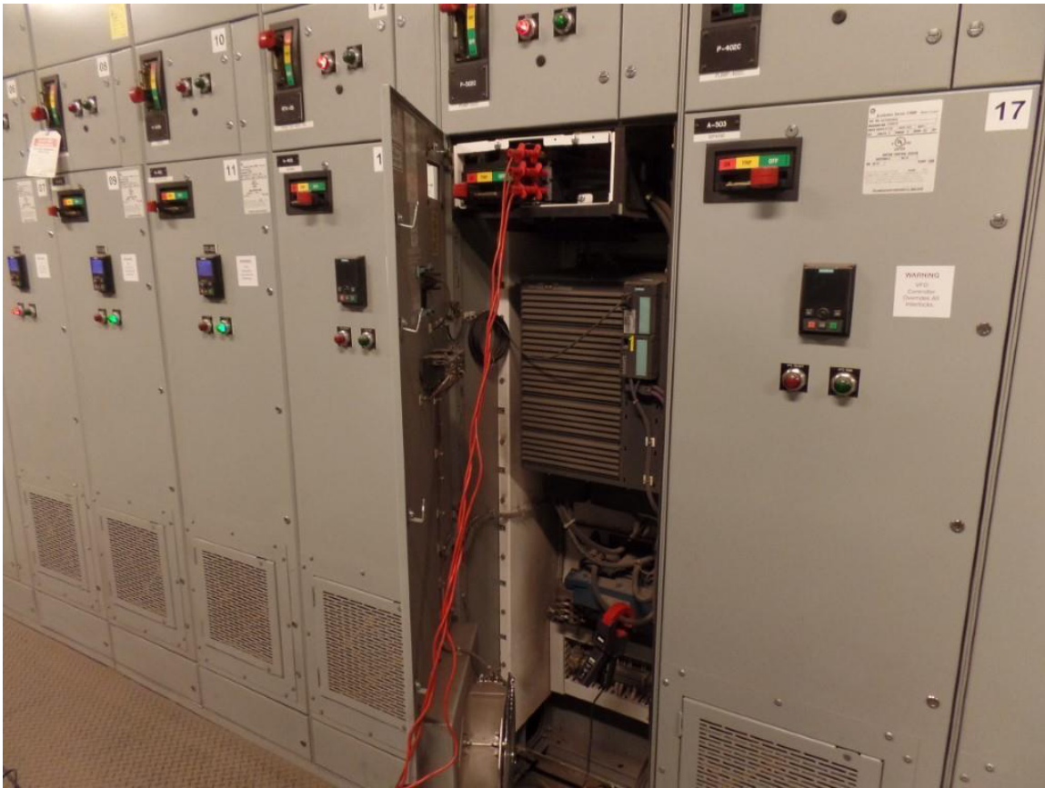
VFD 5043 Pump 502 Voltage Probe and Current Clamp Connections
