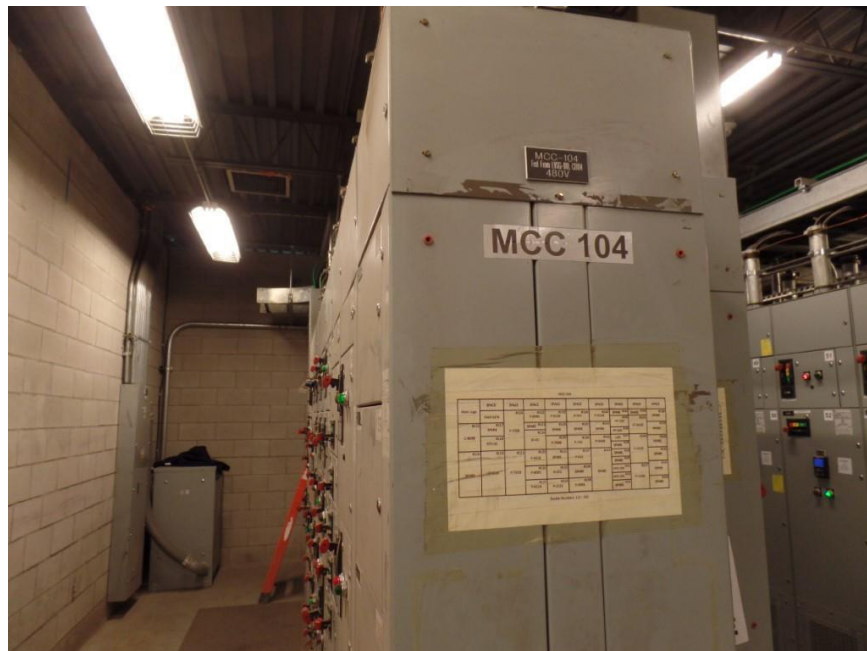
MCC 104 End View
