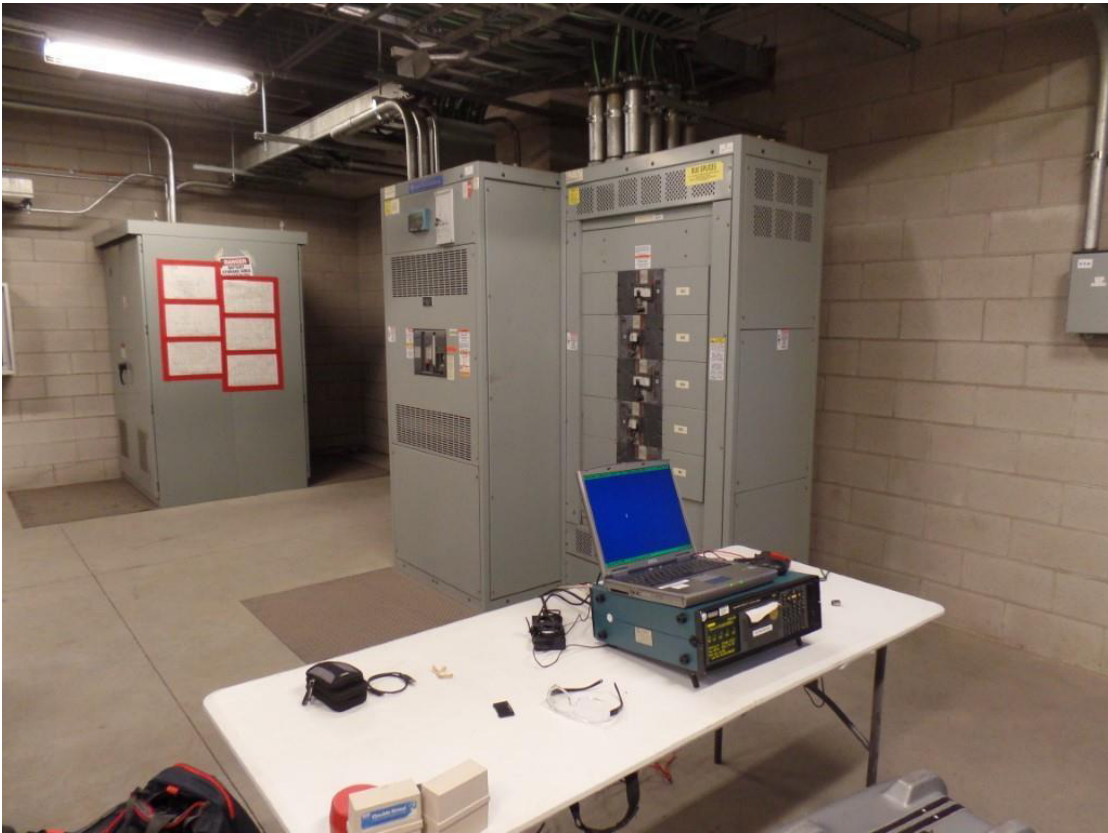
Main Distribution Panel Test Setup
