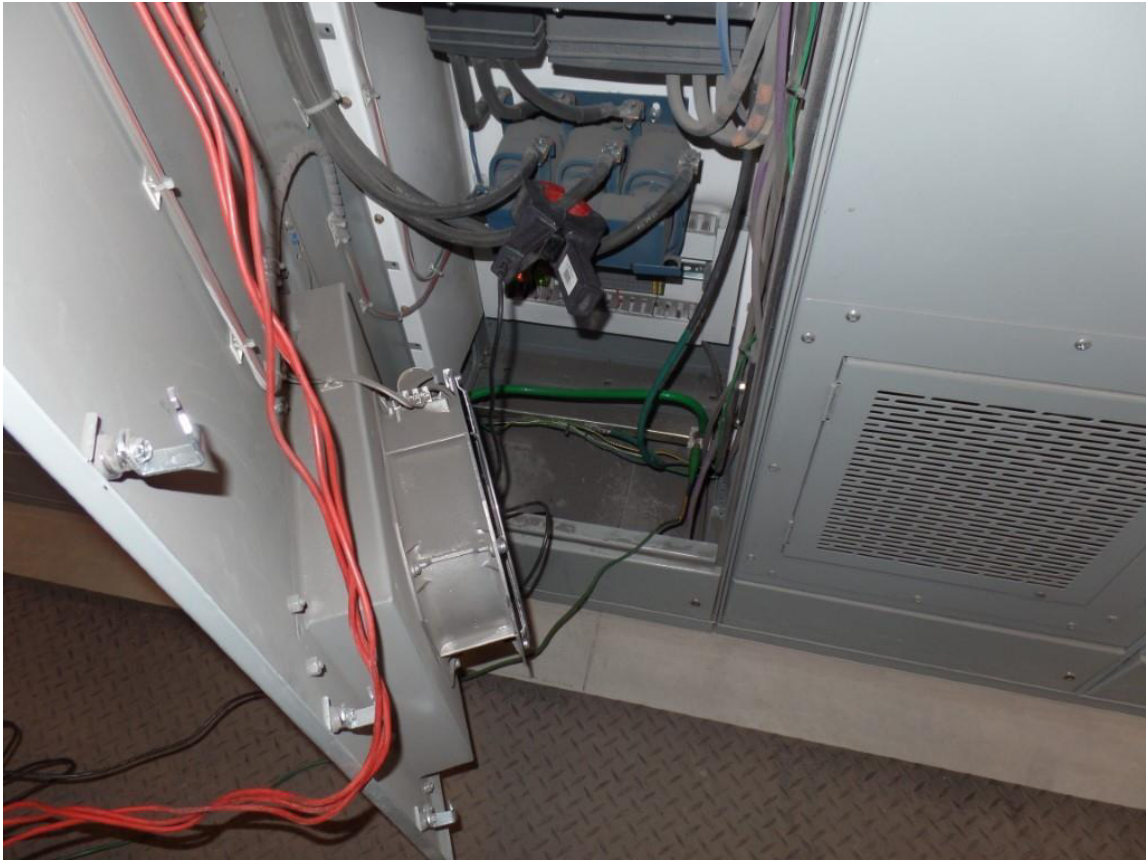
VFD 2057A Pump 211A Current Clamp Connection
