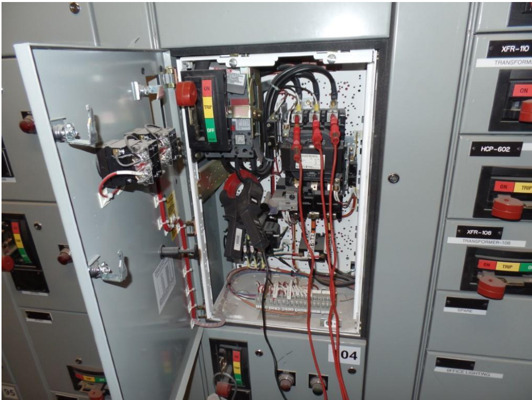
Voltage and current clamp connections for monitoring Pump 201B
