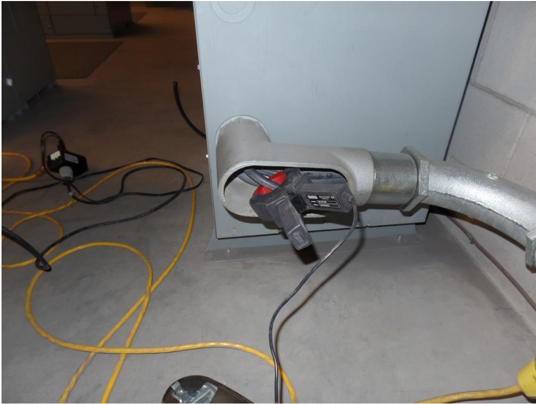
Current Clamp on Phase C on Power Panel PP-105
