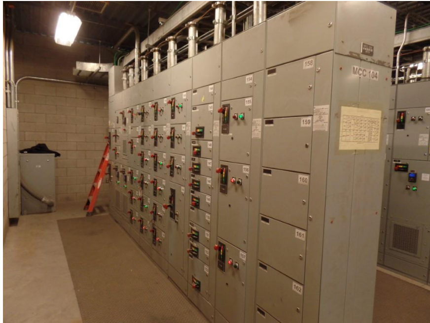
MCC 104 – 10 vertical columns
