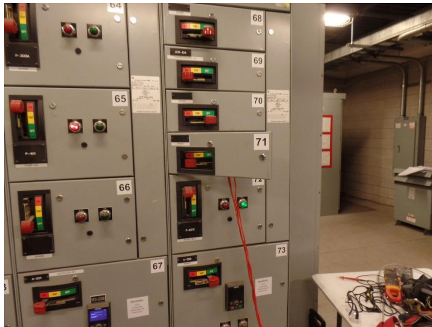
Spare Disconnect in Can #71
