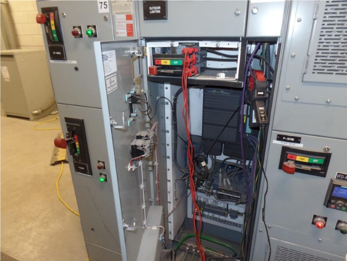
Dranetz Probe connections
