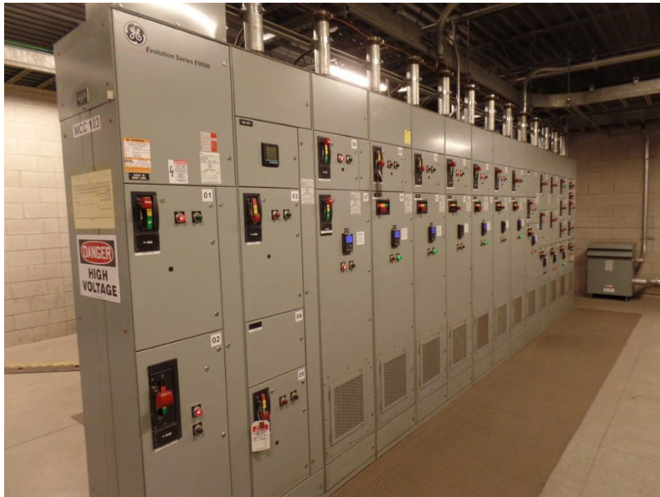
MCC 103 Full View from Left End
