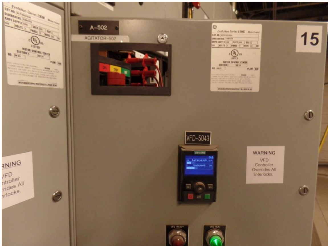
VFD 5043 Pump 502 Name Plates and Display Screen
