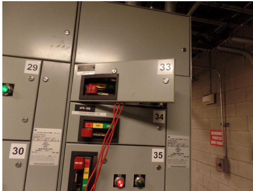
Spare Disconnect on MCC 103 in Can #33
