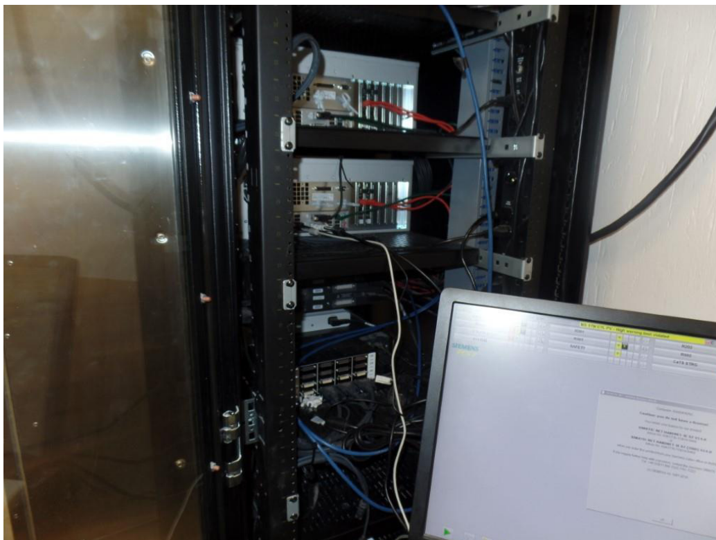
IT/Telecom Rack Equipment
