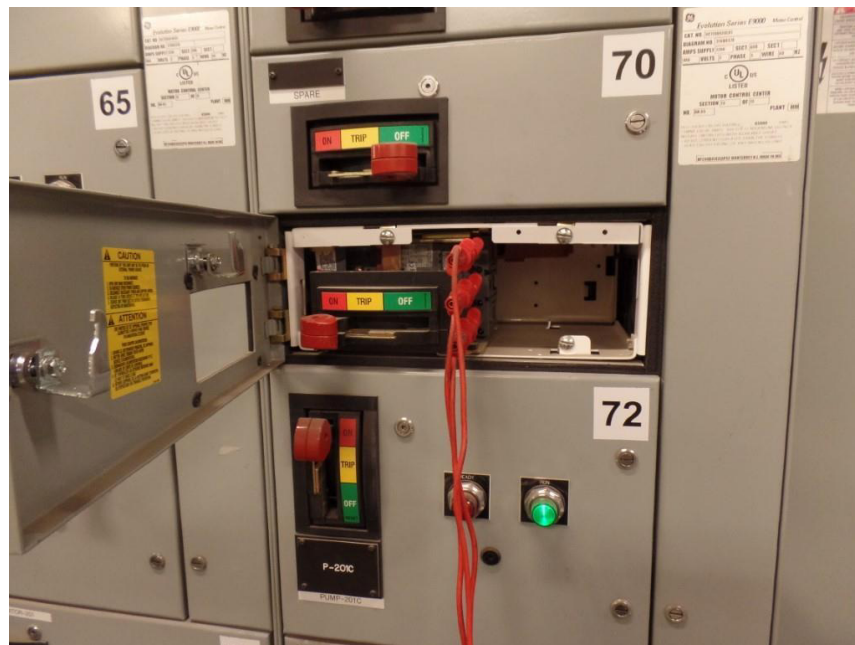
Spare Disconnect in Can #71 Voltage Probe Connections
