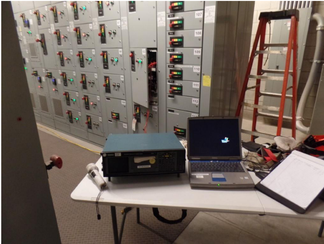
Test setup monitoring Pump 201B
