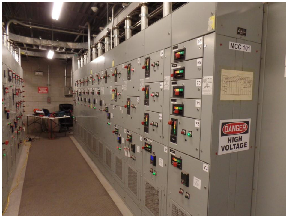
MCC 101 Full View from Right End
