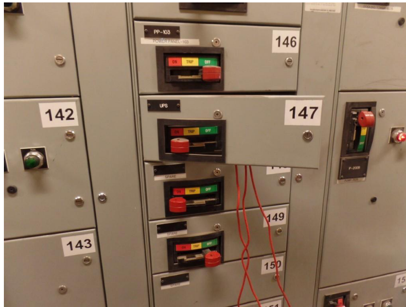
UPS Disconnect Switch
