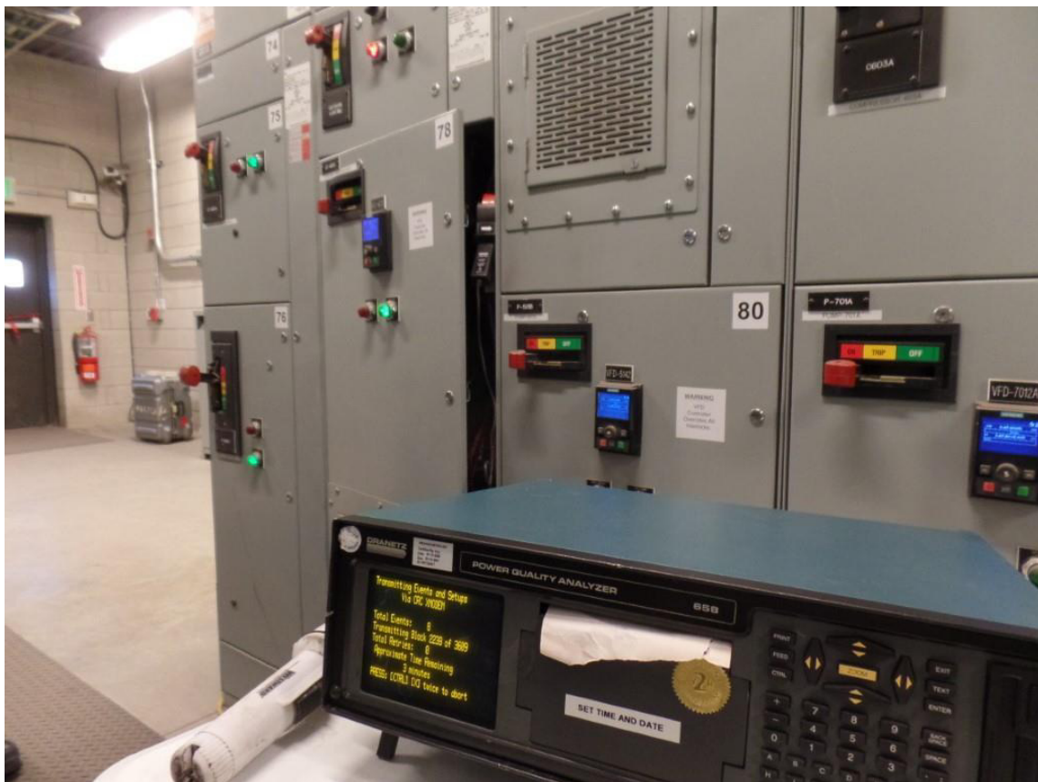
Dranetz connected to VFD 6023 Pump 602C
