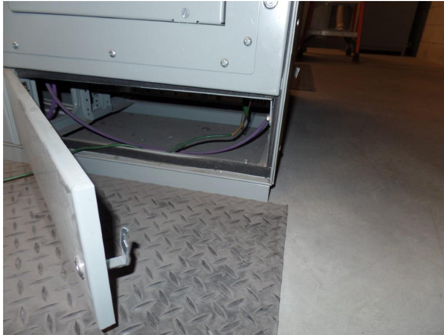
Ground Connection on MCC 103 in Spare Disconnect Can #71
