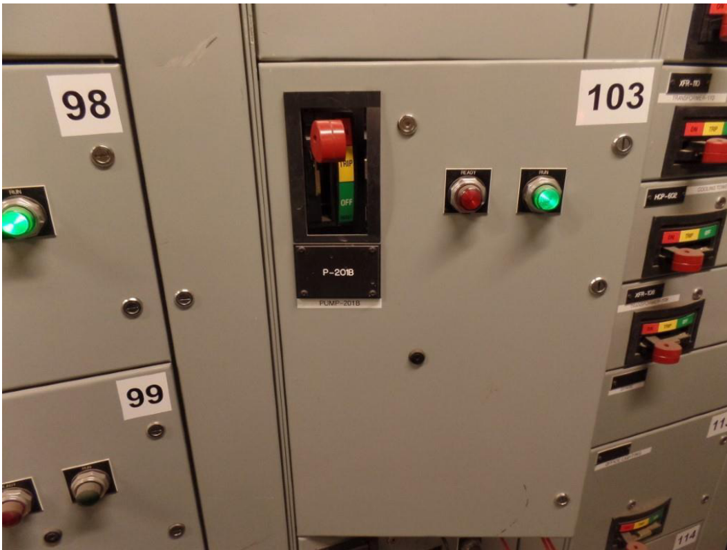
Pump 201B Disconnect Switch
