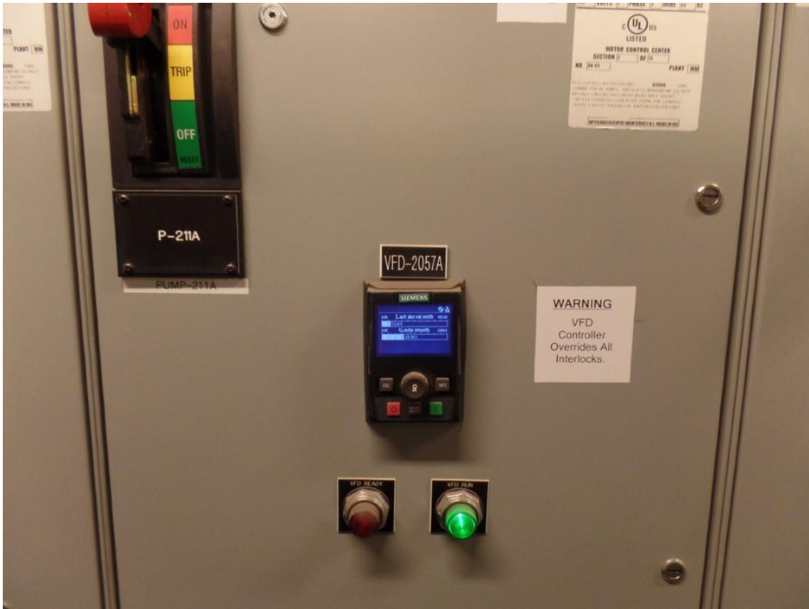
VFD 2057A Pump 211A Name Plates and Display Screen
