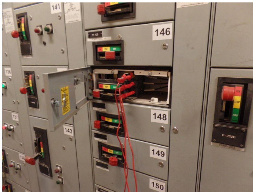
Voltage Probes on UPS Disconnect
