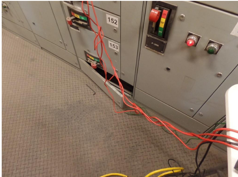
Ground Probe connection for UPS Disconnect Switch
