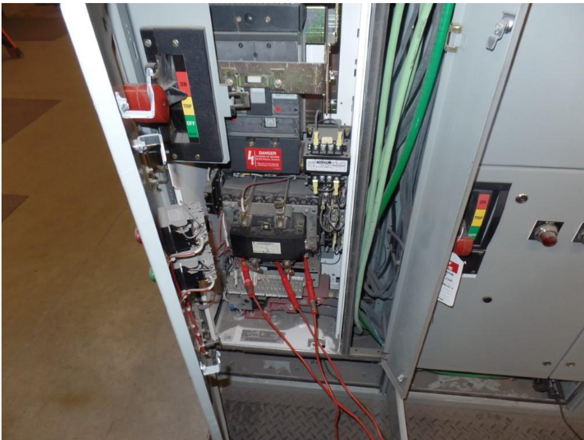
Pump 602B Voltage Probe Connections
