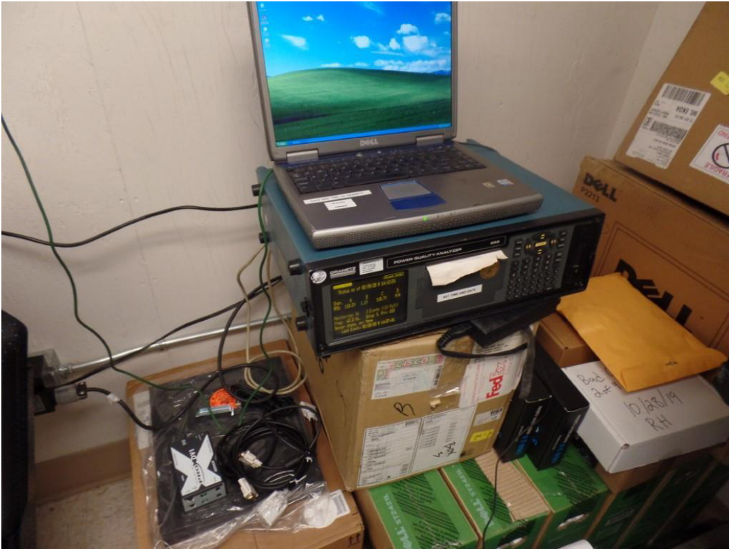
IT/Telecom Power Panel Test Setup
