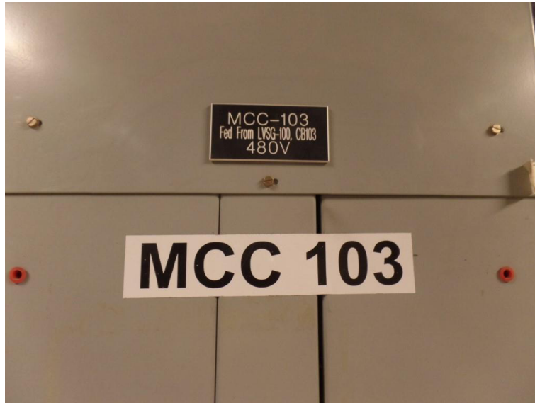
MCC 103 Name Plates
