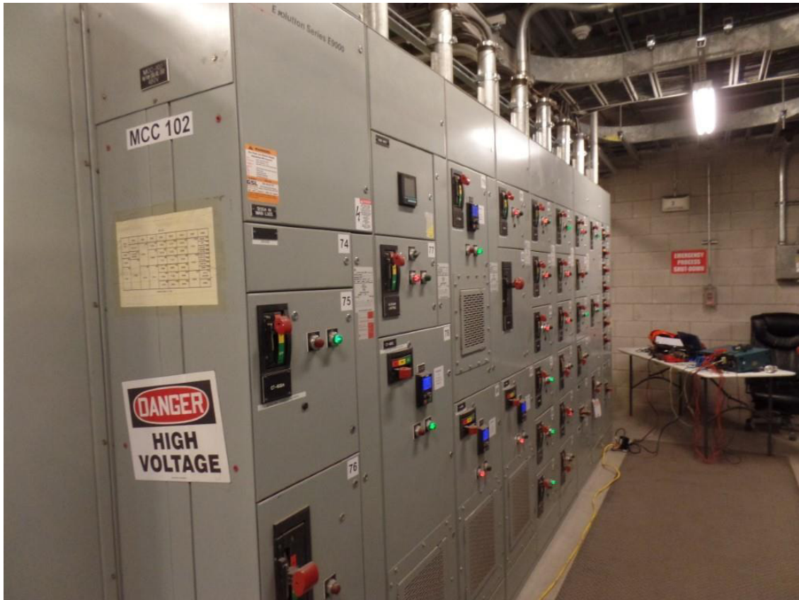
View from end of MCC 102
