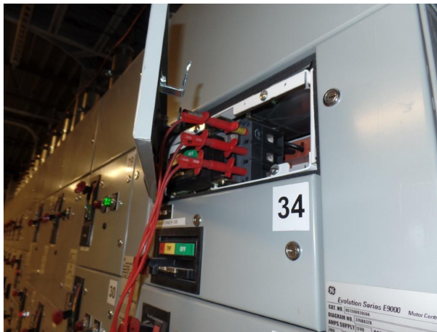
Spare Disconnect on MCC 103 in Can #33 Voltage Probe Connections
