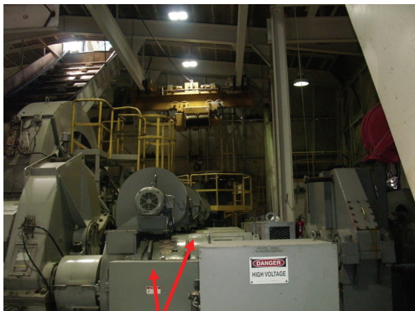
480 V motors, several hundred horsepower
