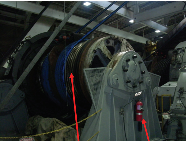
Large Crane Pulleys (note the size of the fire extinguisher)
