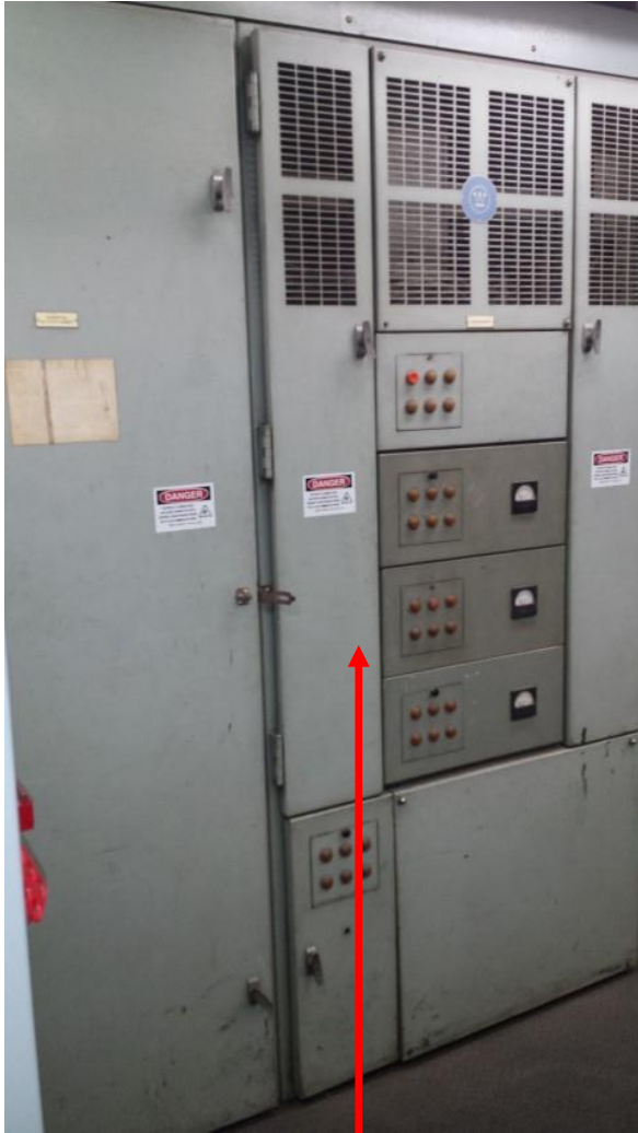
Finishing Mill Drive Cabinet
