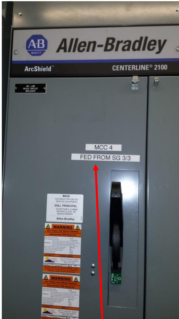
MCC 4 Main Lugs panel
