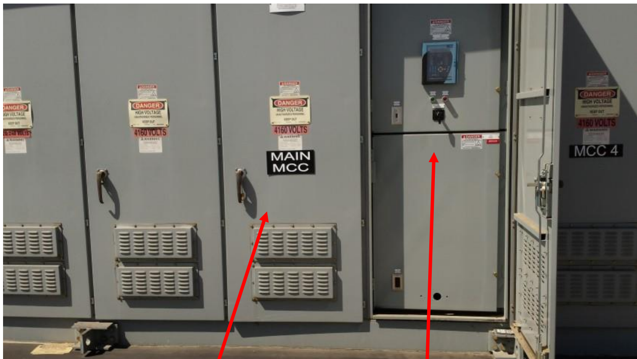
4,160 V Main MCC
